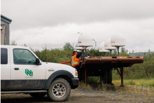
Northwestel technicians installing a series of OneWeb LEO dishes in Inuvik, N.W.T., to rapidly augment local capacity when fire burnt through a fibre line. (Supplied/NorthwesTel)
